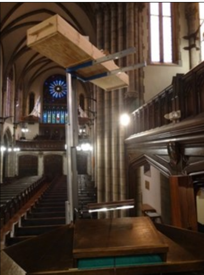
Pipes and other parts are removed with care from the Great division using a hand-cranked lift.
